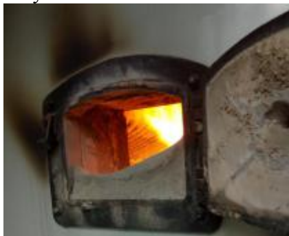
Figure 3 Photo of combustion chamber in the chain boiler(HHO generator installed)
